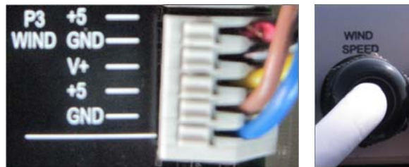
Fig 4-3 Wiring of wind speed sensor
